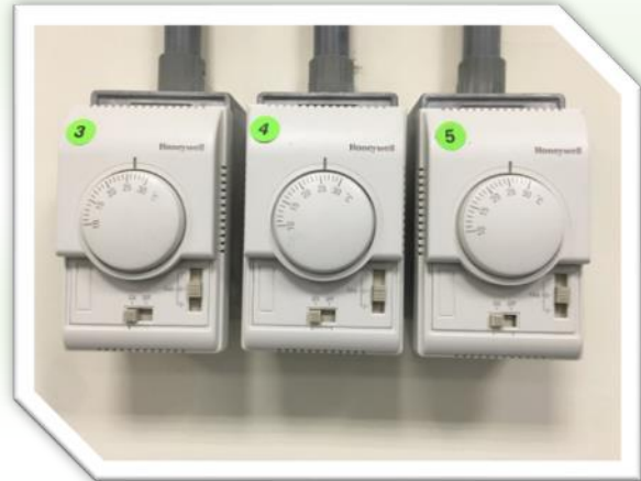
ASRock employs temperature-regulated air conditioning systems.
